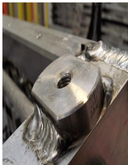
(SPS024) Clamp for Rusted Knobs (Off-Site Repair)
